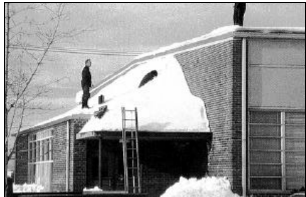
Figure 4. The peak snow load of this drift was 130 psf. The ground snow load at the time was 20 psf, and the snow load on the upper roof was 15 psf.
