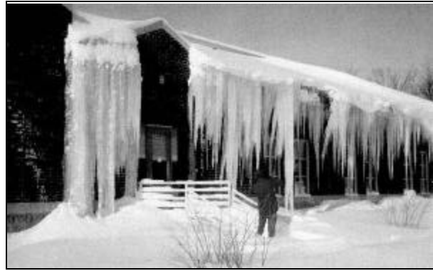
Figure 11. Severe icings developed all along the eaves of this facility.
