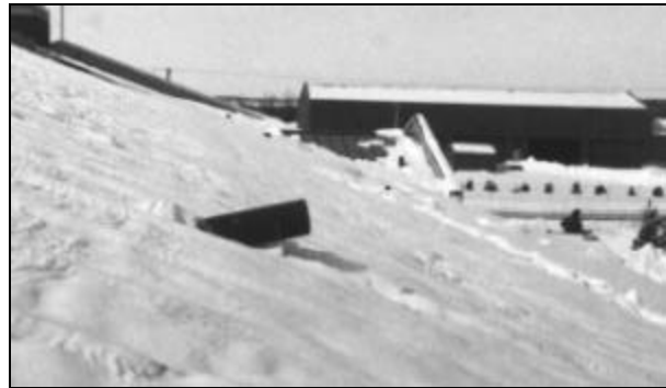
Figure 8. Plumbing vent displaced by snow creeping down a slippery metal roof.
