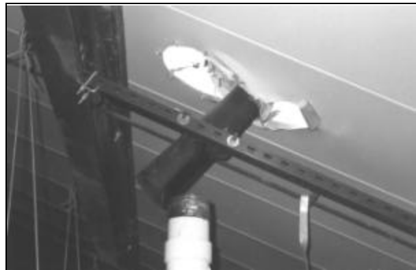
Figure 9. Tear in metal roof caused by plumbing vent displacement shown in Fig. 8.
