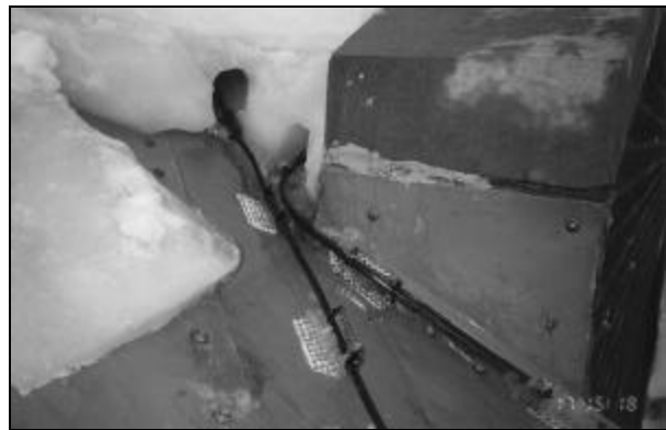
Figure 12. Electric heaters can create tunnels, which limit ponding behind ice dams on roofs.
