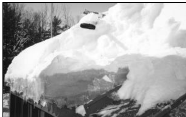
Figure 2. This large ice dam caused this metal roof to leak at its eaves.
